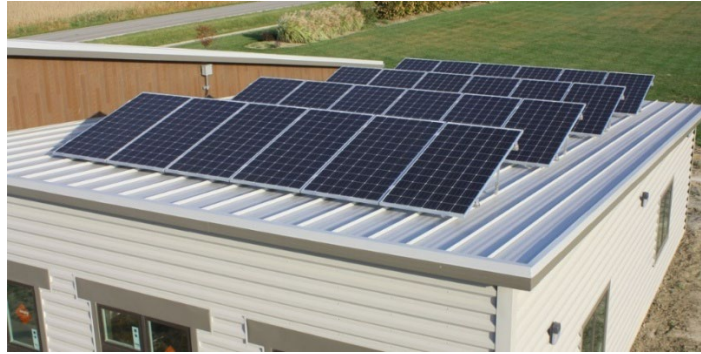
Example of a Solar Conversion System, Structure-Mounted
