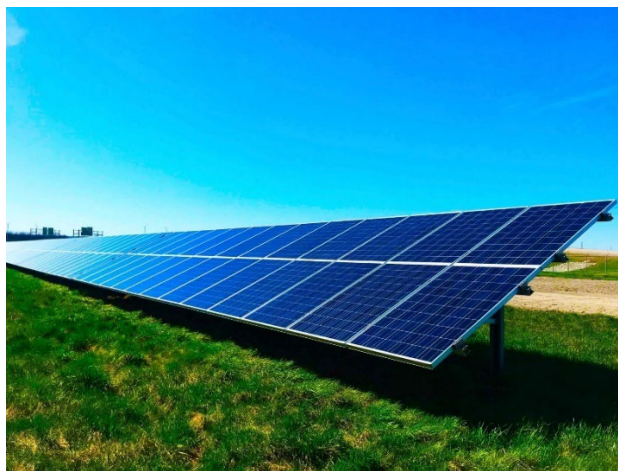
Example of a Solar Conversion System, Ground-Mounted
